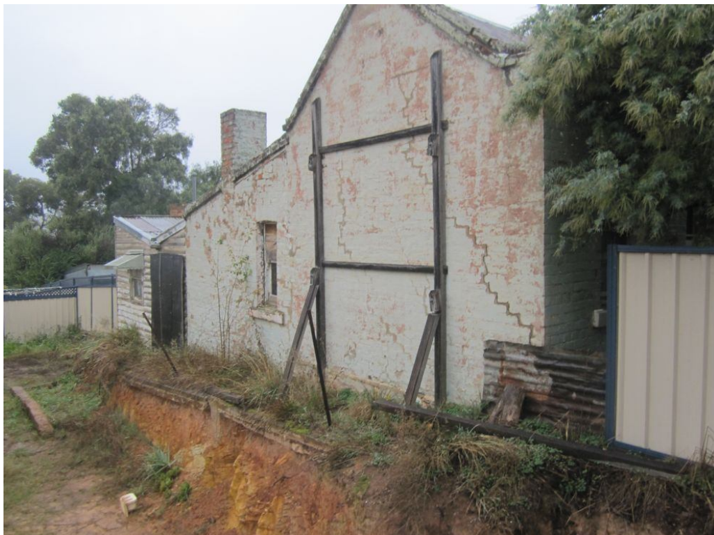
Figure 10 Excavation on adjacent property made many years ago. This wall has not demonstrated any marked rotation.
