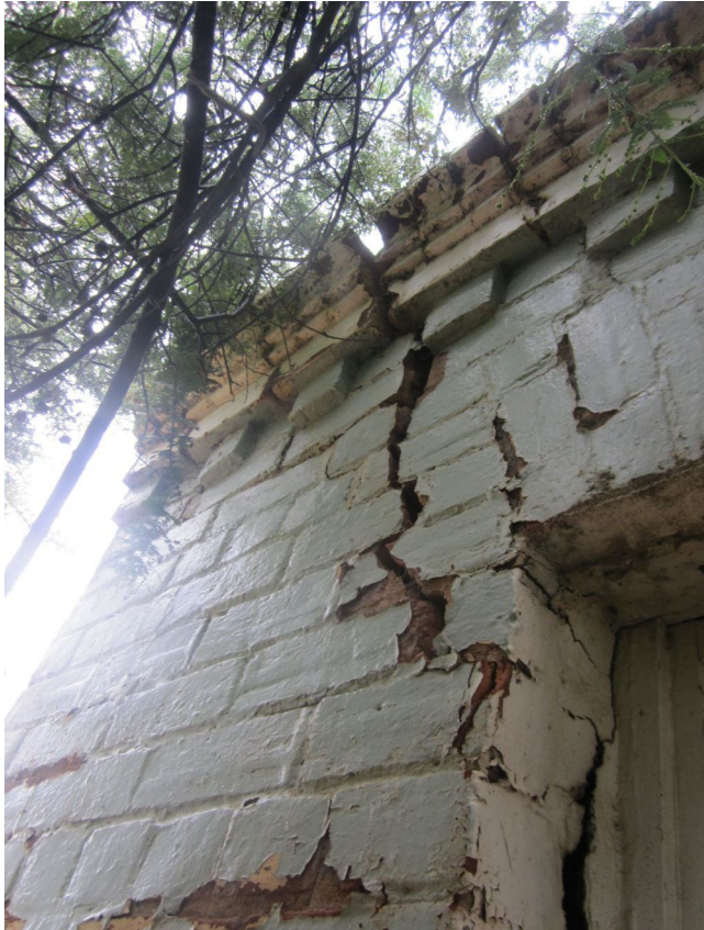
Figure 11 This is the worst external cracking, above the window nearest the tree and corner of the building, the weakest part of the structure. Some minor rebuilding is now required to rectify the alignment, and to replace damaged bricks. Note elaborate parapet detailing.
